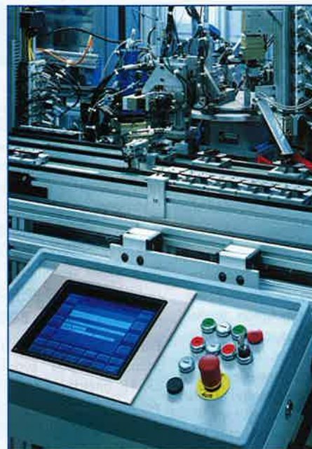
Increased interconnectivity between autonomous devices and systems allows different machines to operate independently and increases flexibility. REF: GAM104
